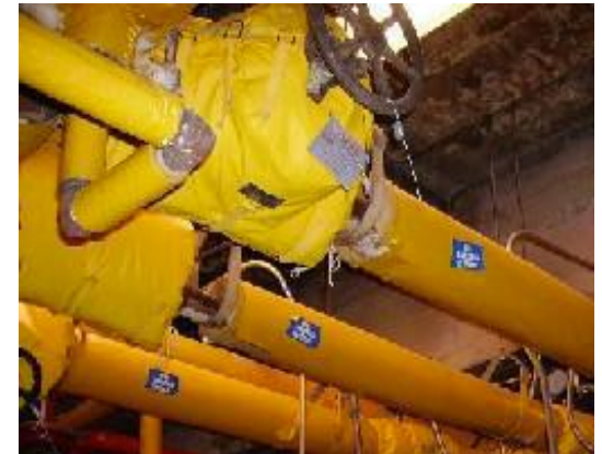
Proper insulation on pipes, valves, and fittings
