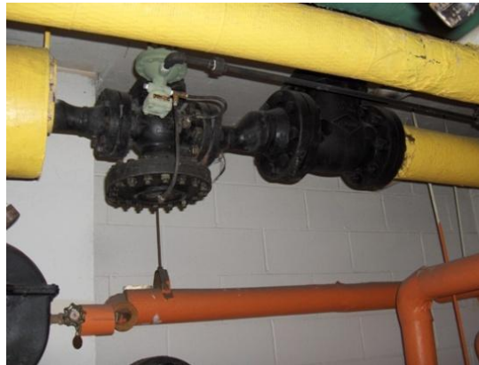
Missing insulation on valves/fittings
