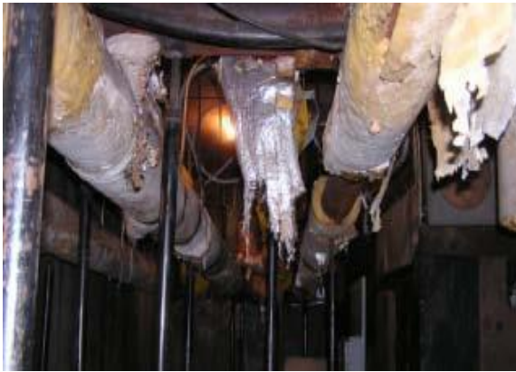
Poorly maintained insulation
