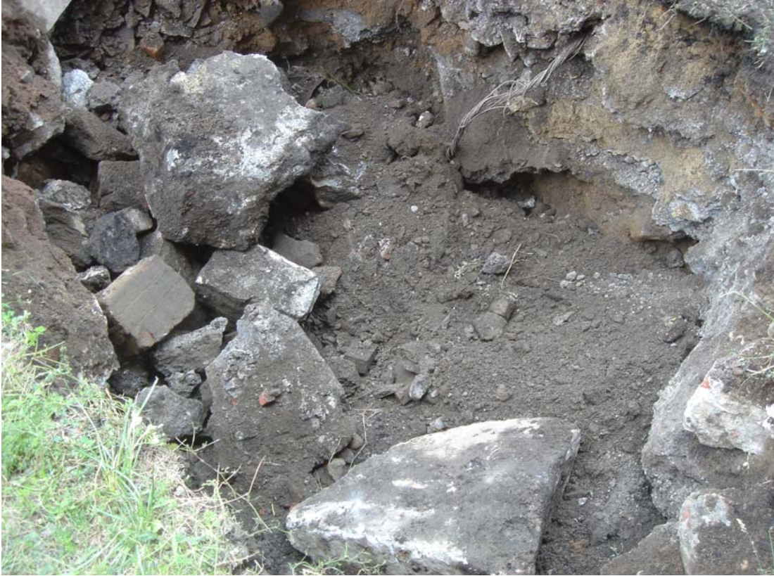
5. Large concrete fragments and boulders at test pit PMW-2 near UST on the north side of the building.
