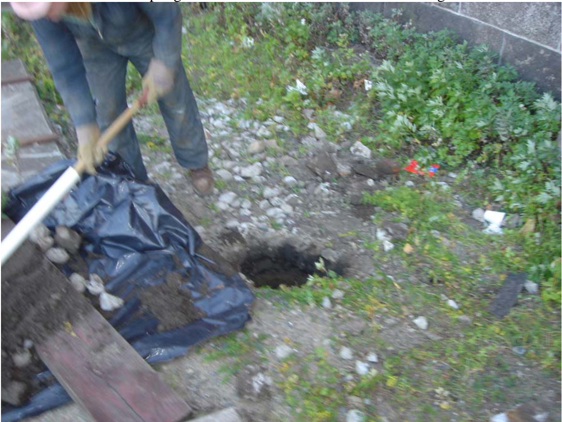
8. Hand augering soil boring S-1 on the north side of the building.
