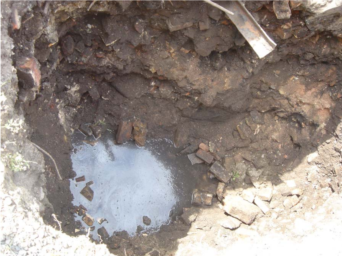
4. Numerous bricks and debris at test pit PBL-8, groundwater at approximately 9.5 ft.
