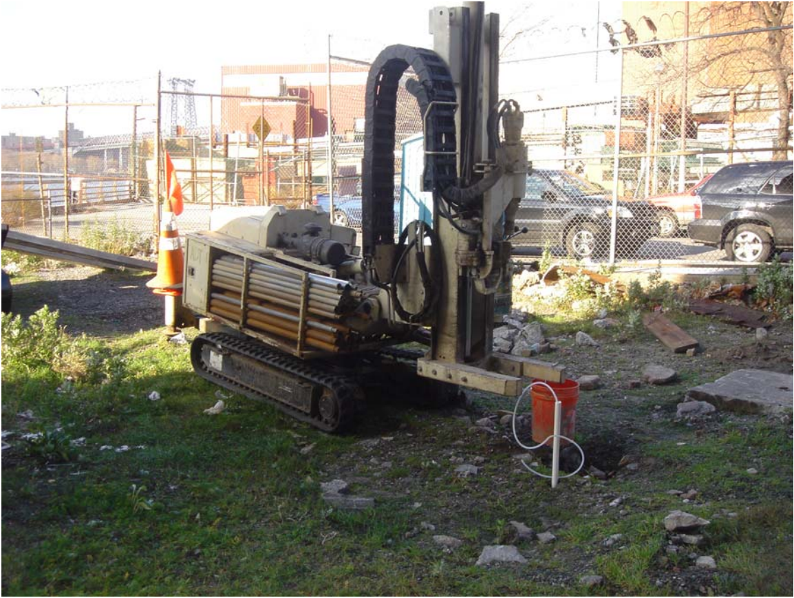
7. Installation and sampling of GW-1 on the north side of the building.
