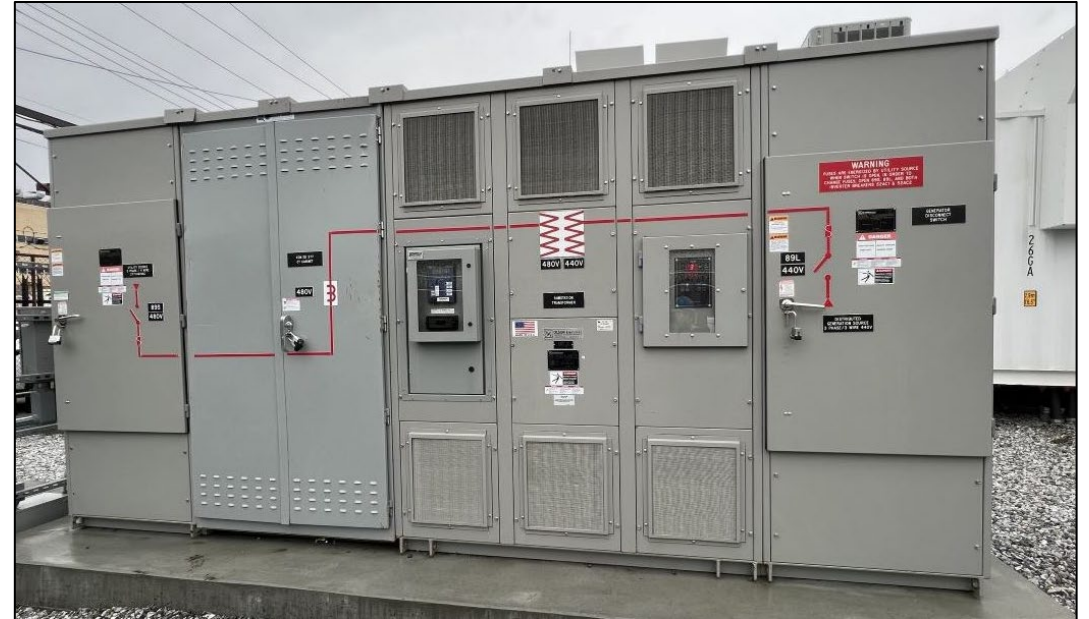
Battery Energy Storage System in Woodside, Queens
