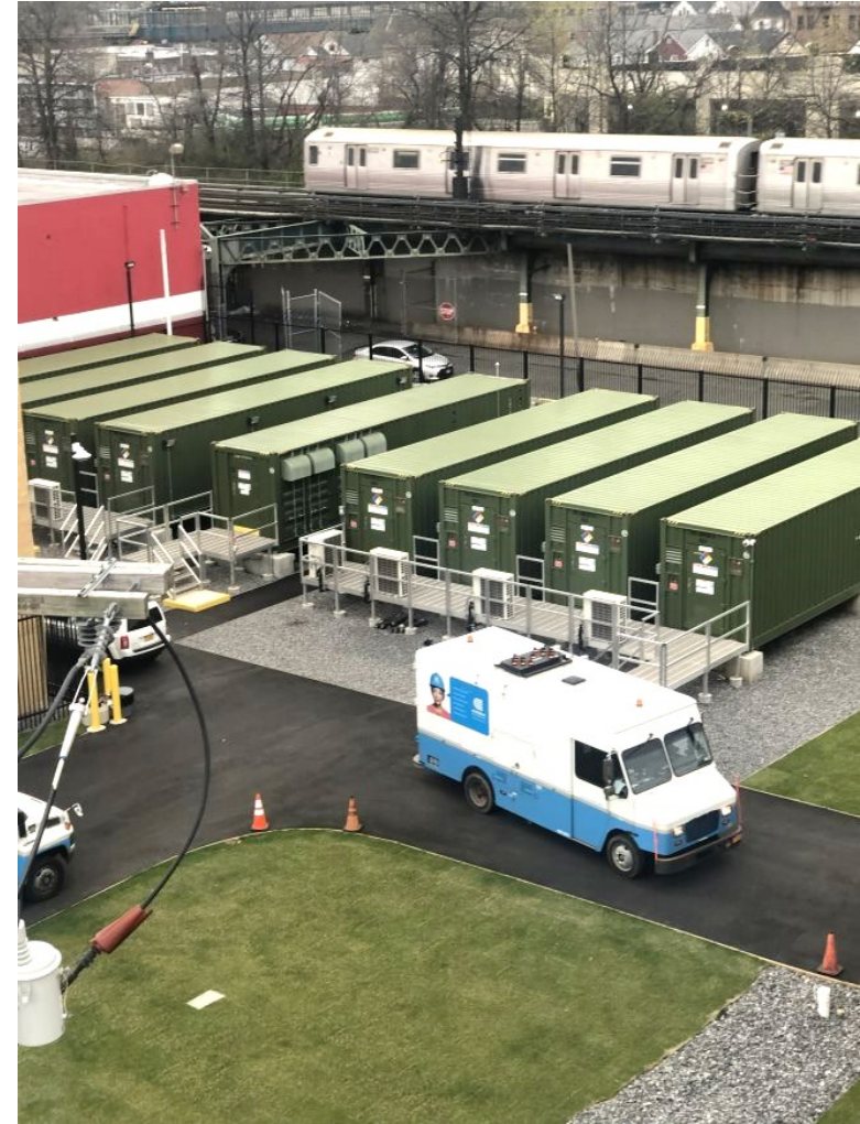
Battery Energy Storage System in Ozone Park, Queens
