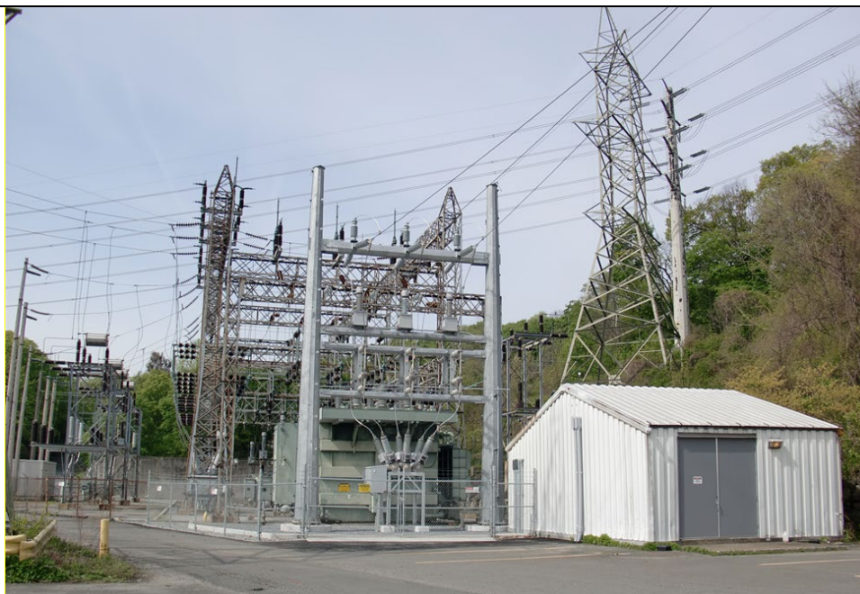
Figure 1. View of the Lovett 138kV substation yard with the control house located in the foreground to the right (white building).
